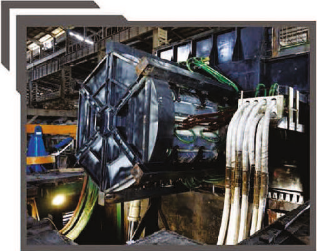
40 Ton capacity Induction Furnace Crucible
